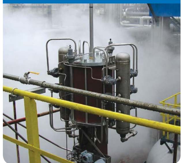
SVI II AP on steam conditioning valve
